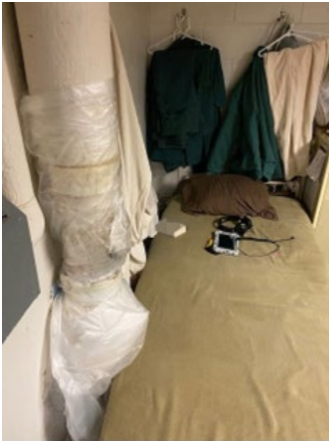
Condition of Pipes and Their Proximity to Inmate Beds in a Basement Housing Floor Source: OIG, January 2023 (Book Title Blurred in Image)
