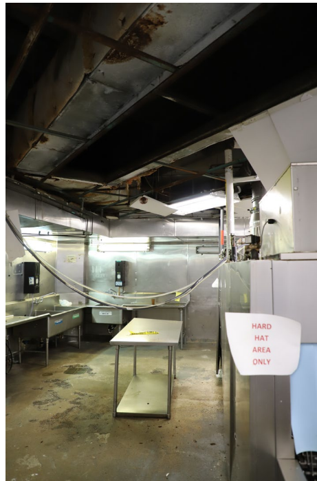
The Food Services area in complete disrepair, including exposed and corroded rebar in the ceiling, MCC New York.
