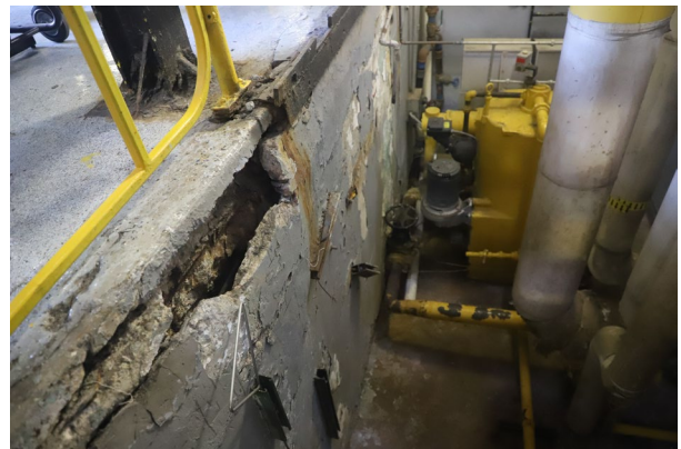
Cracking and separation in the powerhouse floor, where the boilers are located, FCI Terminal Island. Source: OIG, April 2022
